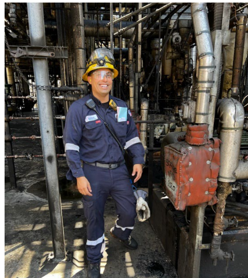
Hot Oil Pump Training
