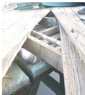
Dock A Mainwalk Framing Structure Worn to fair condition
