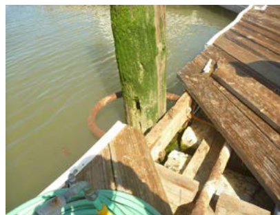
Dock D Mainwalk Framing Structure Dry rot observed
