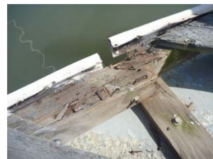
Dock D Finger Framing Structure Broken deck boards and uneven walking surfaces
