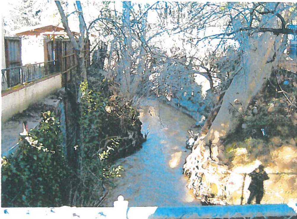
Alhambra Creek downstream of D Street - Large trees 10-15 feet apart constrict channel and limit conveyance.
