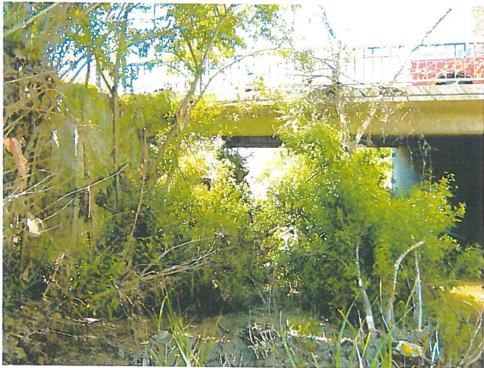
Trees blocking Ward Street Bridge
