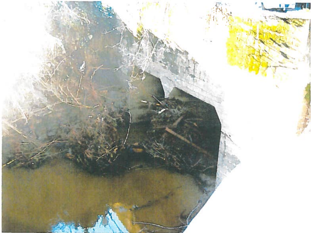
Uprooted tree lodged in culvert blocking flow and limiting conveyance
