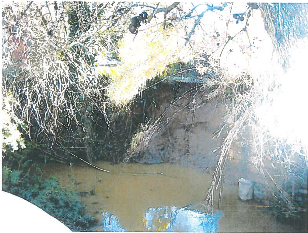
Retaining wall failure on east bank upstream of Brown Street culverts
