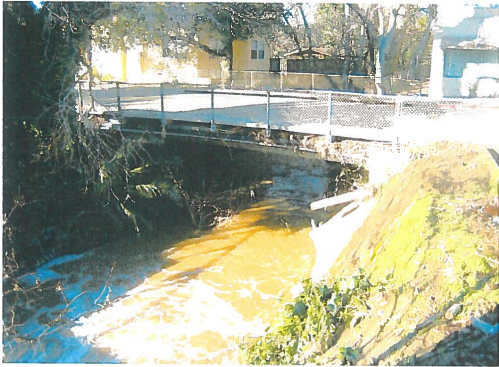
Alhambra Creek Channel - D Street Bridge is narrower than upstream channel section. Debris trapped in drainage slots.
