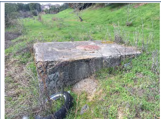
Manhole cover associated with partially exposed concrete storm drain pipe
